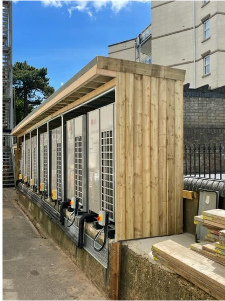
VRF Units Housing with cantilever.
